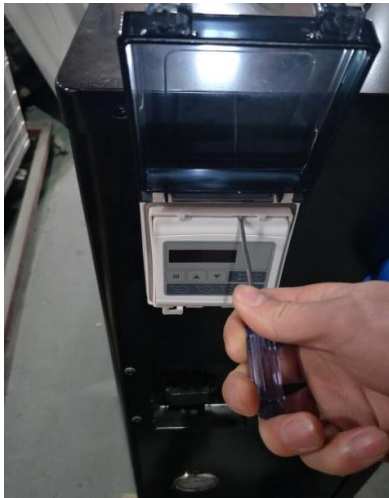
Pic. 1a (inverter)
