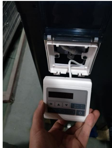
Pic. 2a (inverter)
